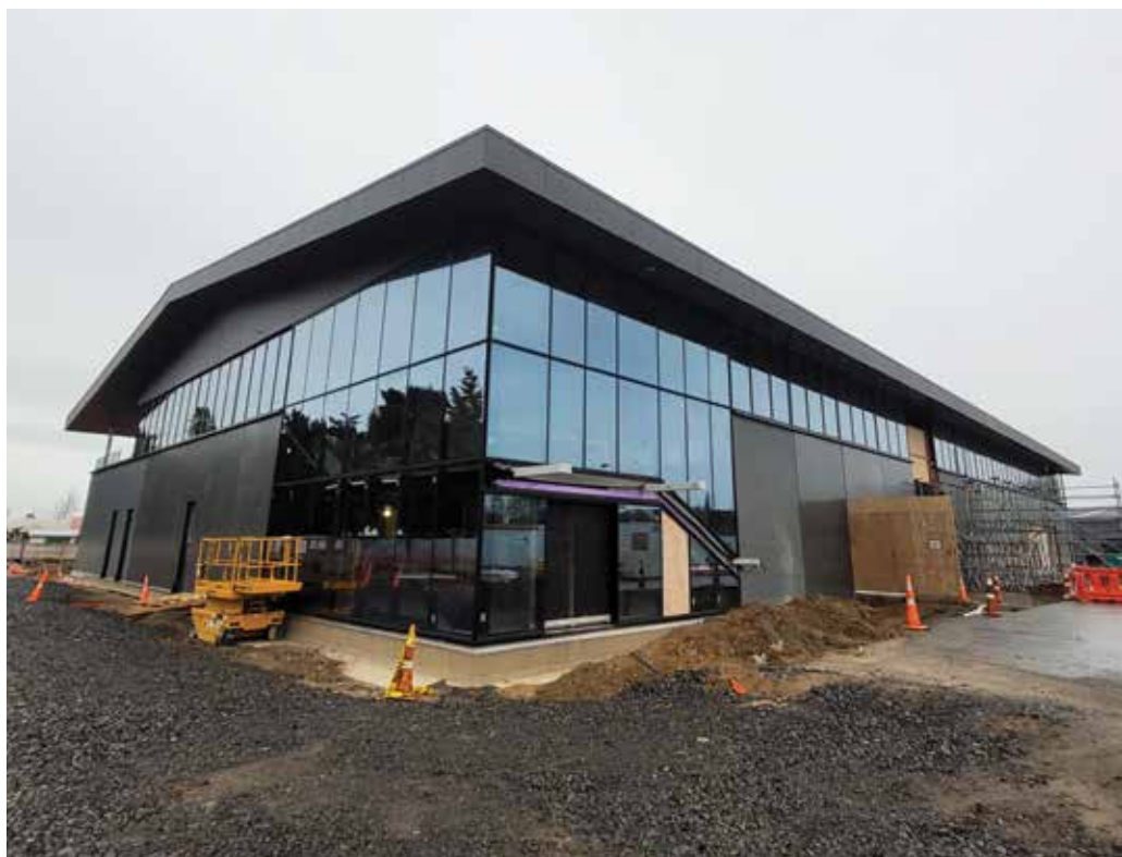
NIWA’s new Hamilton facility on the University of Waikato campus is scheduled for completion in mid-2023. [Blanton Benjamin, Foster Construction]
