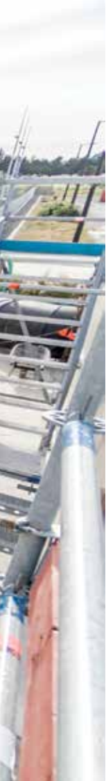
Members of NIWA's Board and Executive inspecting the recirculating aquaculture tanks under construction at the Northland Aquaculture Centre. [Lana Young]
