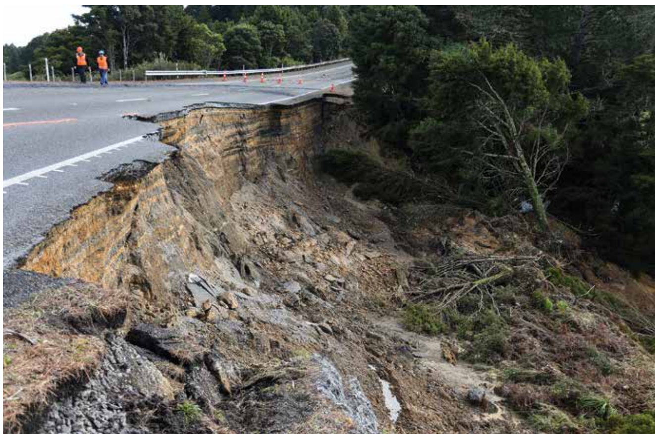
A slip closes State Highway 1 north of Towai. (Michael Cunningham, Northern Advocate)
