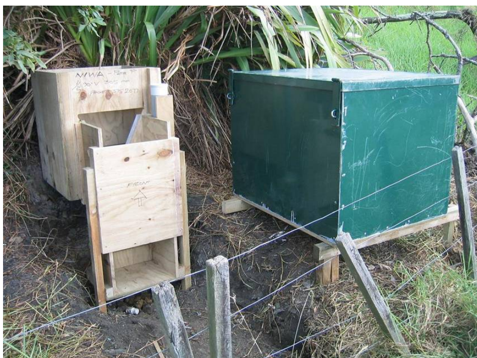
Figure 3.3 SH18 @ Westgate: weir, instrumentation for water level measurement and automatic sampler cabinet
