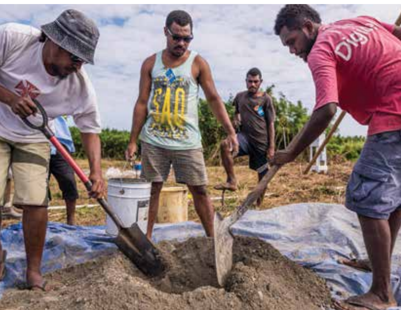
Project Coordinator Sam Tapo (centre) prepares the concrete – mixed 'island style' on a tarpaulin. (Dave Allen)
