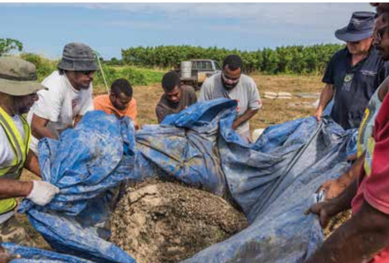
Mixing concrete – island style. The concrete foundations for the weather station will help the instruments hold up to extreme winds that are likely in future cyclones. (Dave Allen)
