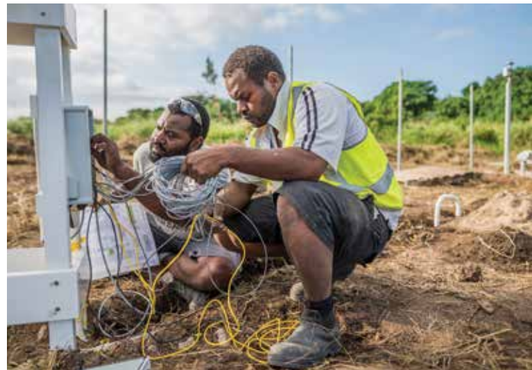
VMGD Technicians Jeremy Bani (left) and Loic Jimmy work on a colour-coded patchwork of cabling to the Stevenson Screen – a standardised housing for instruments to measure air temperature, humidity and atmospheric pressure. (Dave Allen)
