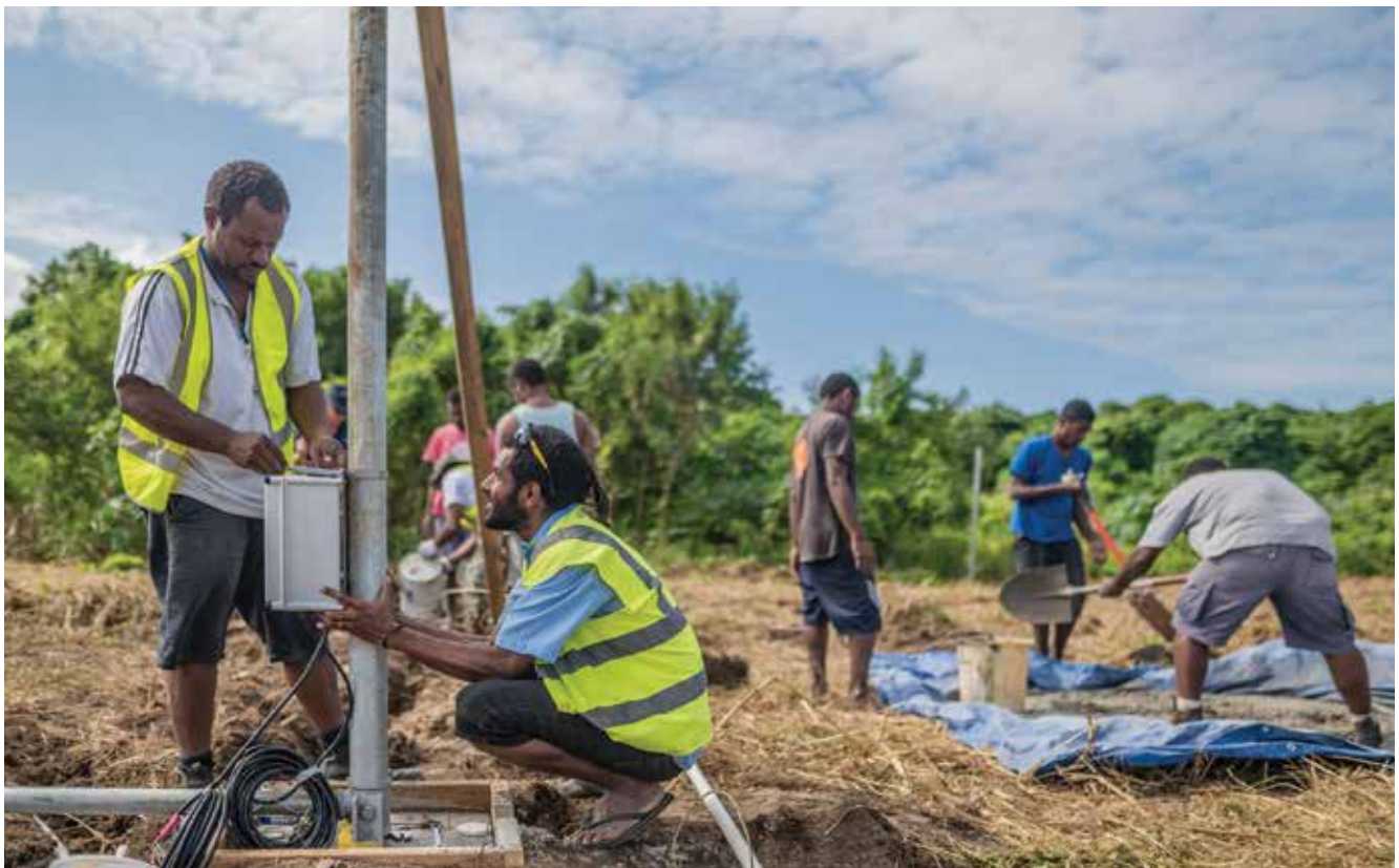
VMGD Technician Jeremy Bani (Left) and local Observation Officer Bradley Bani install cables on the weather station mast. (Dave Allen)
