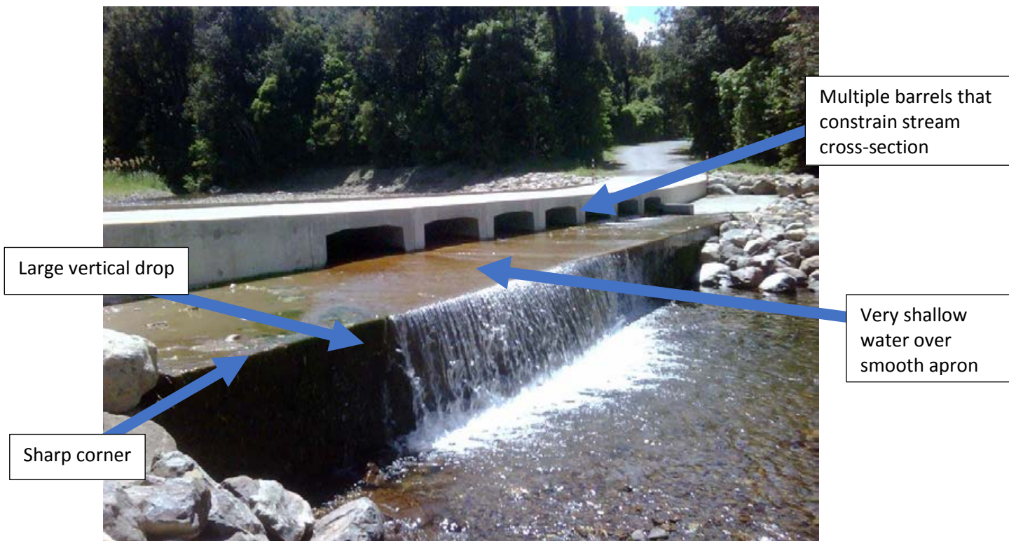
Figure E-18: An example of a drift-deck ford. This is a significant barrier to fish due to the large fall height on the downstream side of the structure. Passage may also be impeded by the sharp corner on the edge of the apron, shallow water, and high water velocities during high flow.
