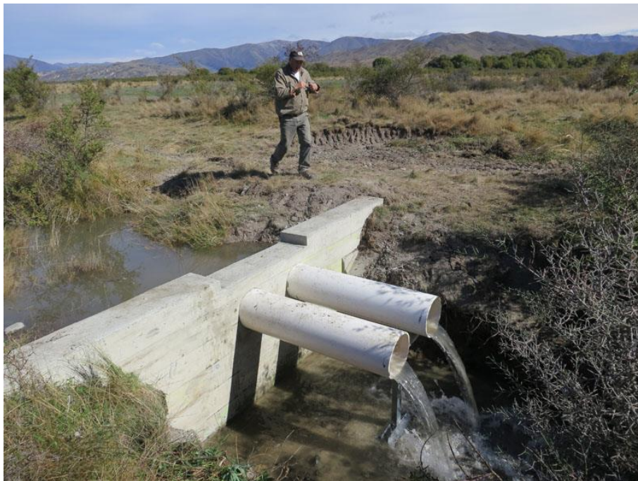
Figure 6-4: Built barrier installed in an unnamed spring of the Ahuriri. The objective was to prevent trout accessing a key lowland longjaw galaxias stronghold in the MacKenzie Basin, Canterbury. Credit: Dean Nelson (DOC).
