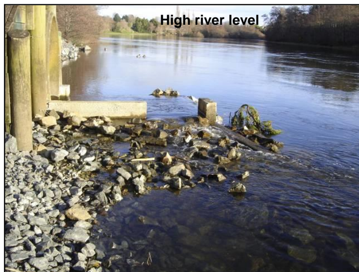
Figure 5-2: Example of a concrete rock ramp below a culvert that is oriented perpendicular to the downstream water body. A receiving pool has been added to the base of the culvert to direct the ramp downstream along the river margin. This provides the foundations for a low gradient sloping ramp.
