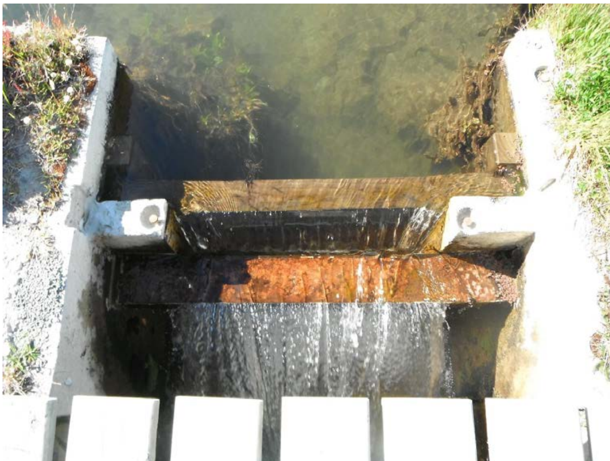
Figure 6-13: Wooden slots on the Fraser Spring built barrier. Credit: Sjaan Bowie.
