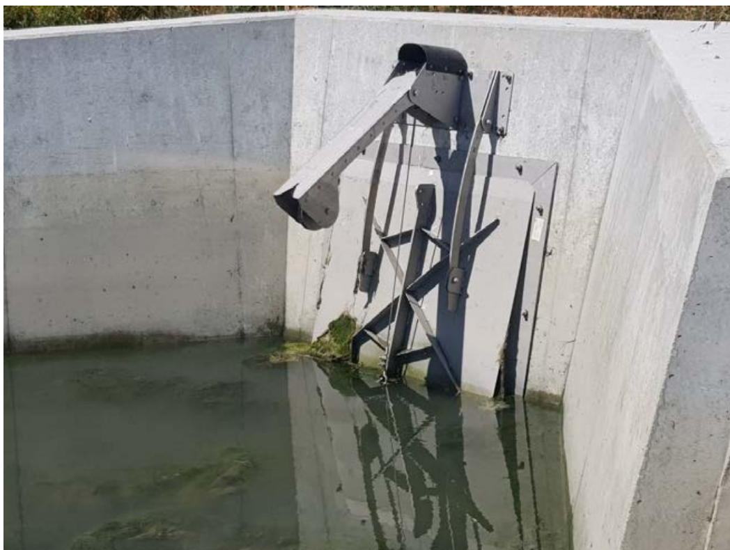
Figure 4-19: Example of a self-regulating tide gate installed in Canterbury. The counter weight system holds the tide gate open for longer on the incoming tide. The system can be calibrated to manage the magnitude and duration of the opening to best coincide with critical migration periods, e.g. the incoming tide for whitebait and elvers.
