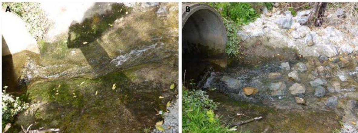
Figure I-3: Culvert apron at Upper Kingston Road. A, unmodified. B, modified using boulders as baffling elements.
