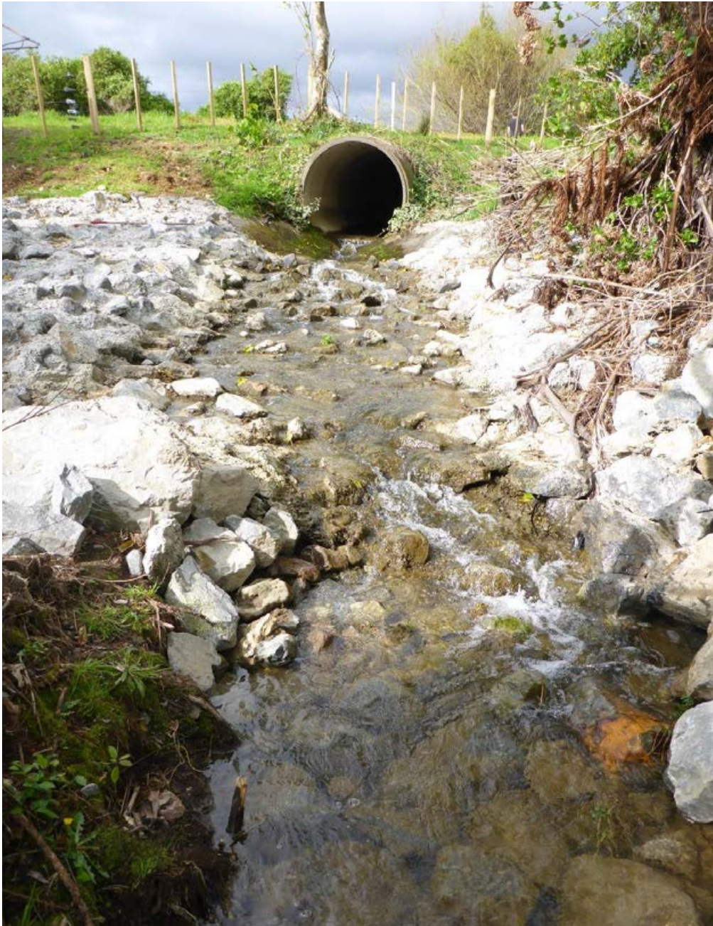
Figure 5-4: An example of a concrete rock ramp below a culvert in the Manawatu-Wanganui region. Concrete is used to prevent water seepage between rocks and is shaped to provide a low flow channel and resting pools to facilitate upstream passage. Photo: Cindy Baker.
