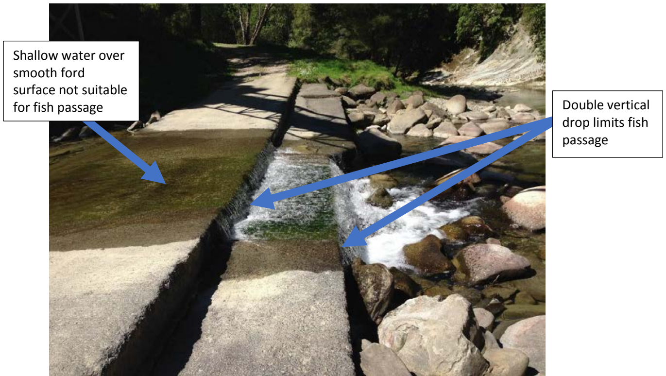
Figure E-20: Example of a ford from the Te Arai River. The fall height at the two steps on the downstream side of the ford makes a complete barrier to swimming fish species. Passage for climbing fish will be impeded by the sharp corners on the steps and shallow water across the ford, but some may access upstream habitats by taking advantage of the wetted margins to climb. Credit: Paul Franklin.
