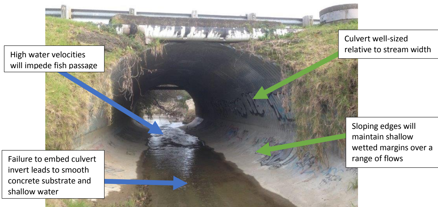
Figure E-23: Culvert well sized relative to stream width, but failure to embed the culvert invert leads to shallow water depths and high water velocity. If this culvert had been embedded so that substrate was retained through the culvert it would have been a good example of how culverts can provide fish passage. Credit: Mark Pennington.
