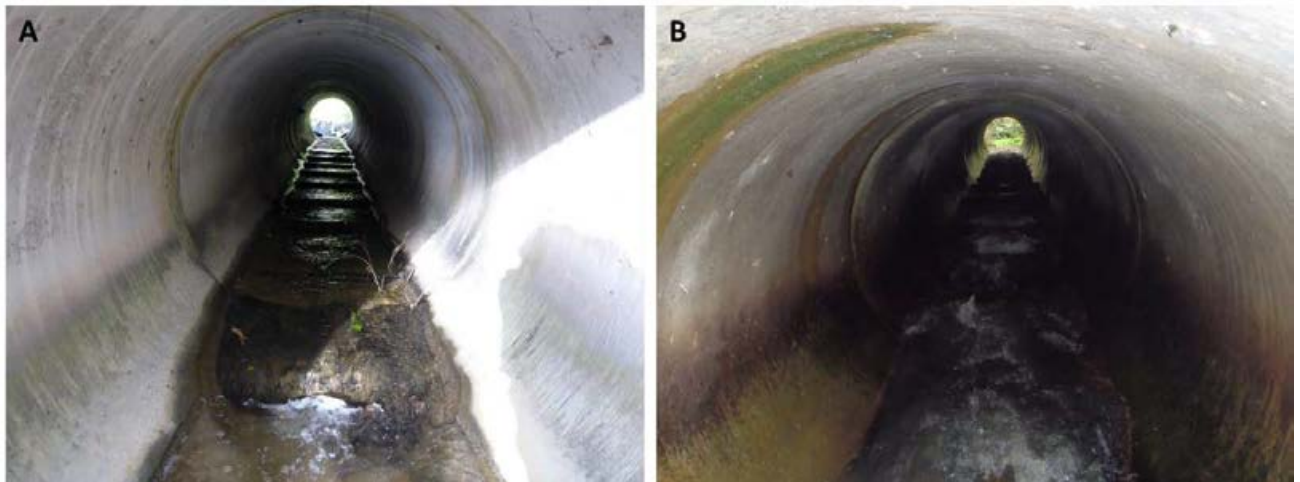
Figure I-2: Culvert under Upper Kingston Road. A, at low flow. B, at high flow.
